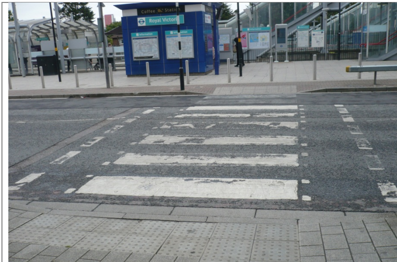
Crossing 32 (Seagull Lane): faded markings & tactiles
