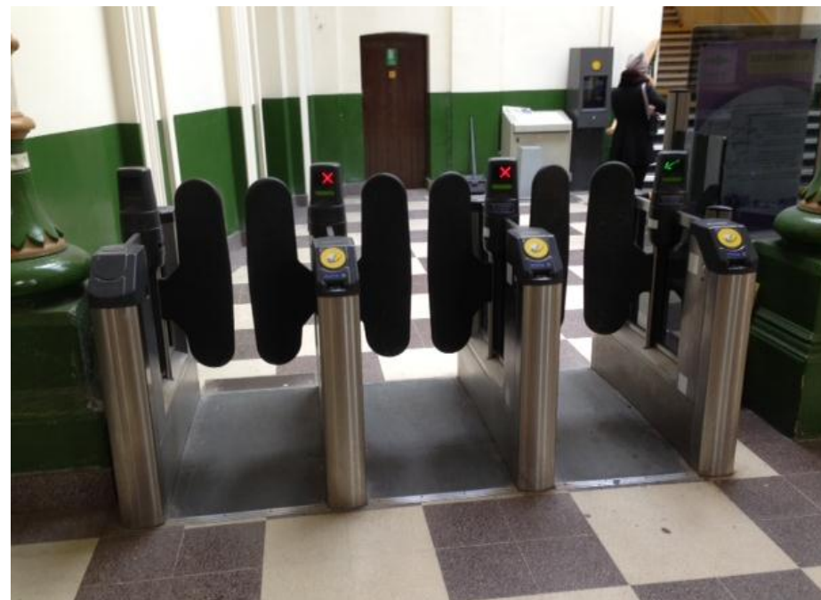
FIGURE 2.2 UTS GATES AT BATTERSEA PARK STATION
