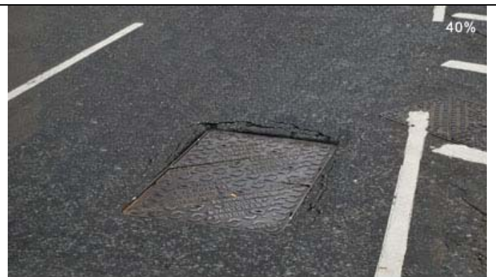
A sinking of the ironwork by 10mm
