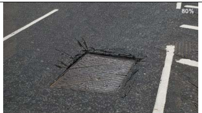
A sinking of the ironwork by 30mm
