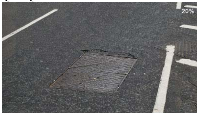
Cracks occurring on the outside of the ironwork
