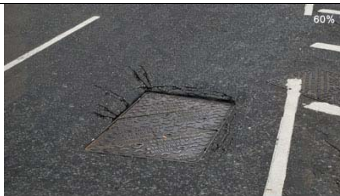
A sinking of the ironwork by 20mm
