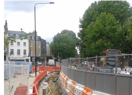
3) Multi Utility Trench
