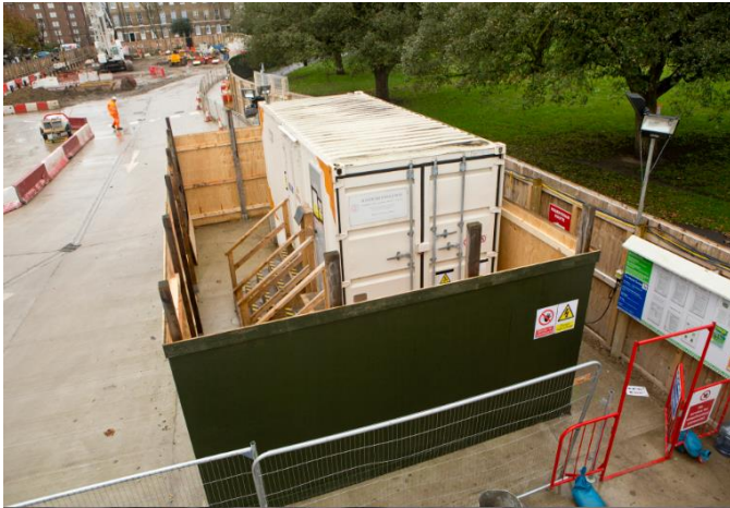
New substation at Kennington Park
