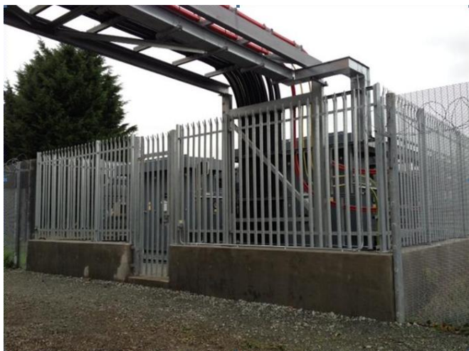
Two 2.5MW Transformer Rectifiers at Hornchurch
