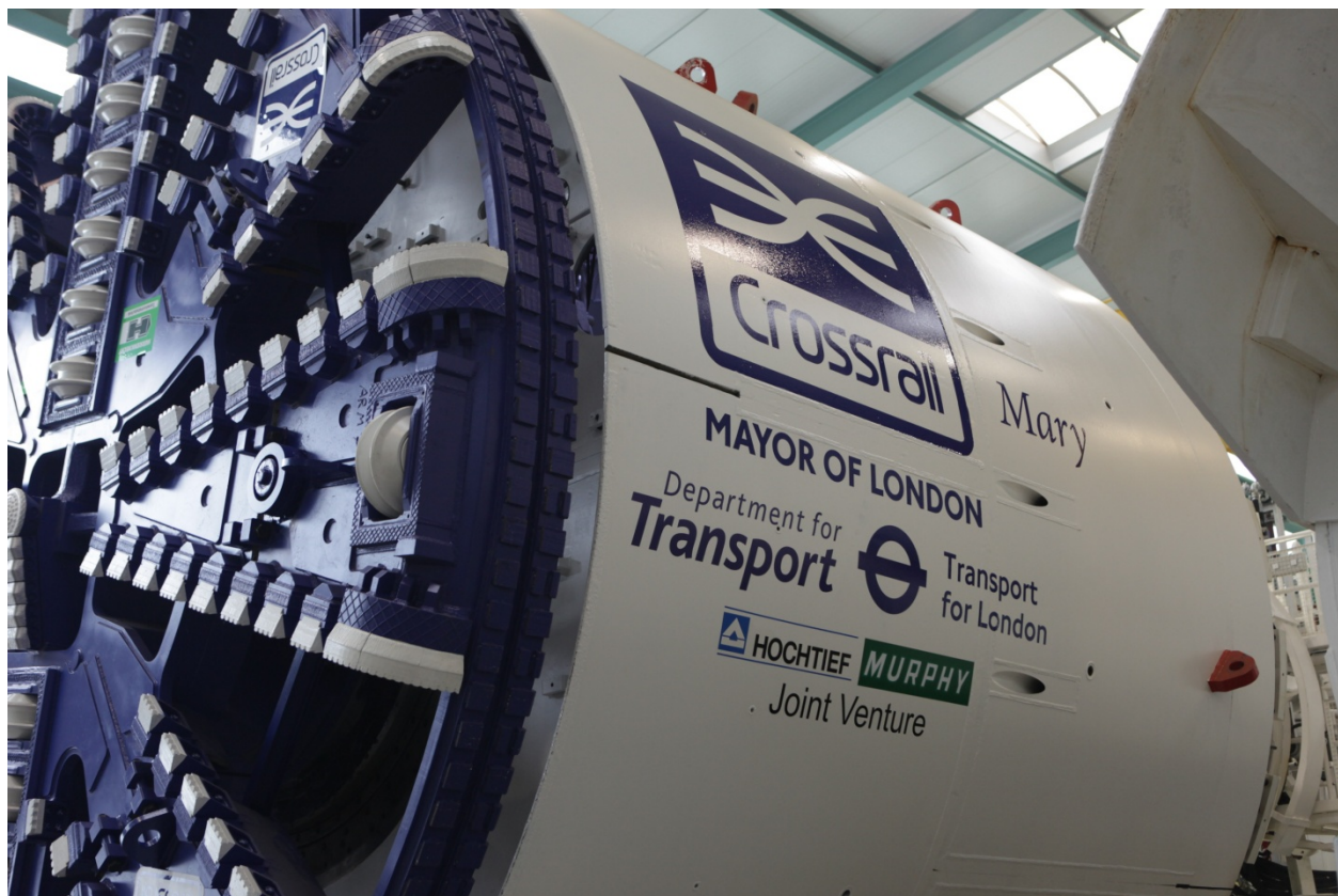
Mary, the 6th tunnel boring machine for Crossrail progressing from Plumstead to North Woolwich
