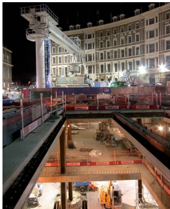
Northern ticket hall site at night © Mike Ashton, Balfour Beatty Civil Engineering Ltd
