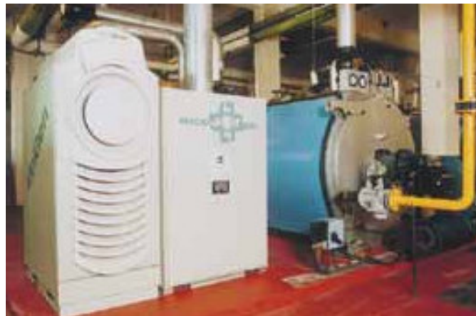
Figure 5.13 – Combined Heat and Power (CHP) plant
