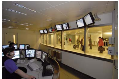
TTH – in operation
