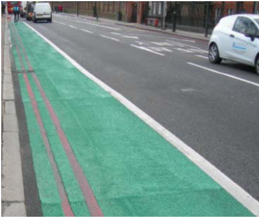
Newly constructed CS5 in use at A202 Camberwell New Road, Eastbound between Brixton Rd and Bolton Crescent
