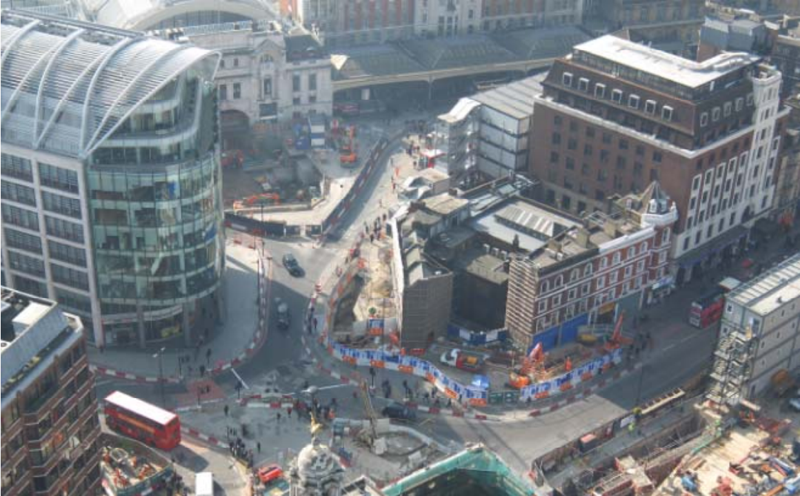
Aerial view of westbound link and south ticket hall worksites at Victoria
