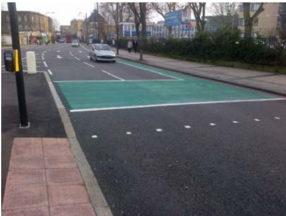
Newly constructed CS5 at A202 Peckham Road at the junction with Kelly Avenue Westbound
