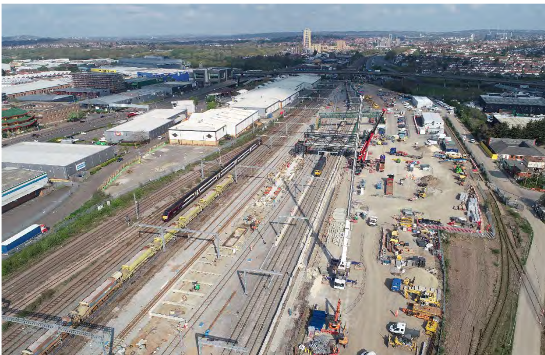
Figure 36: Construction of the new Thameslink Station at Brent Cross West. A station that could be used by West London orbital services in the future
