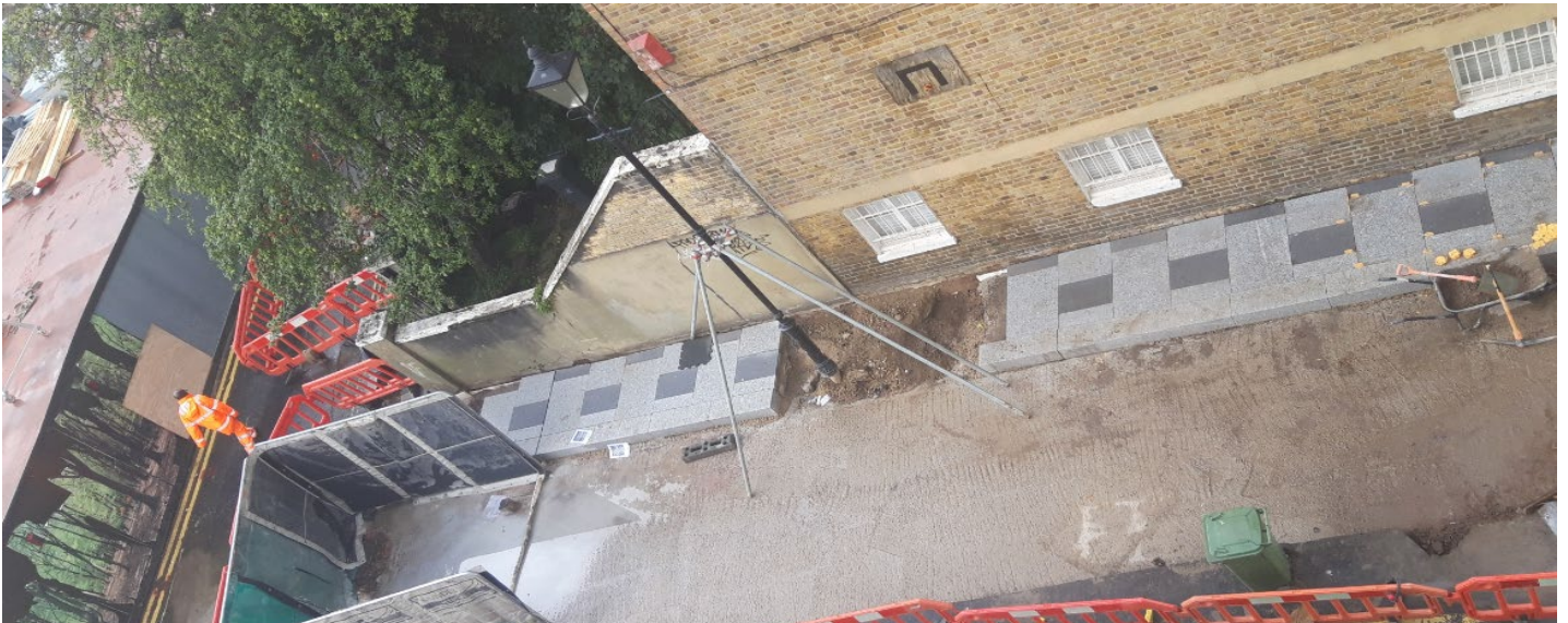
Fig. 3 Hard landscaping works underway - granite paving installation at the NLE Kennington Green site
