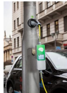
Example of lamp column charging solutions
