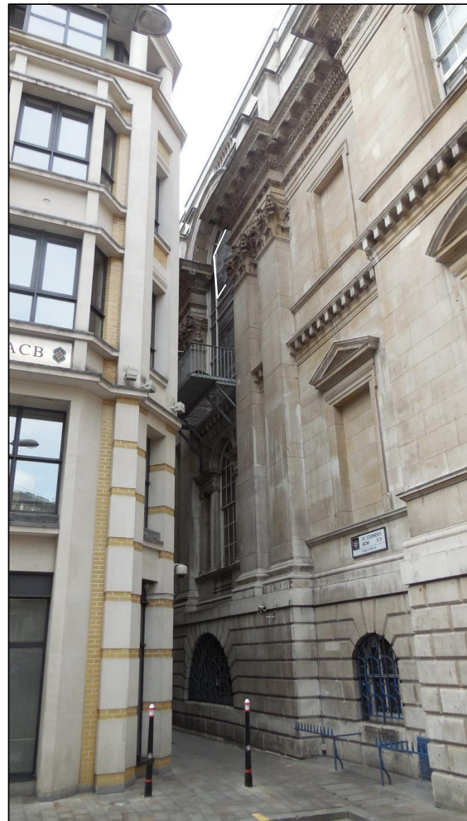
Exterior view of stained glass, with panel to be removed shown in white outline
