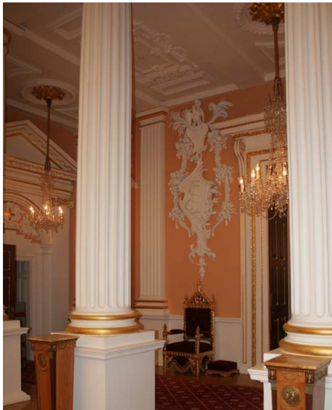
Photo 4: Example of heavy plaster enrichments to walls and ceilings that are at risk of damage due to predicted movement
