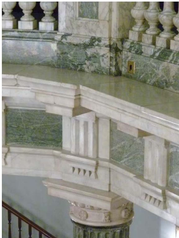
Photo 6: Detail, top of ground floor column to base of first floor column, foyer balcony
