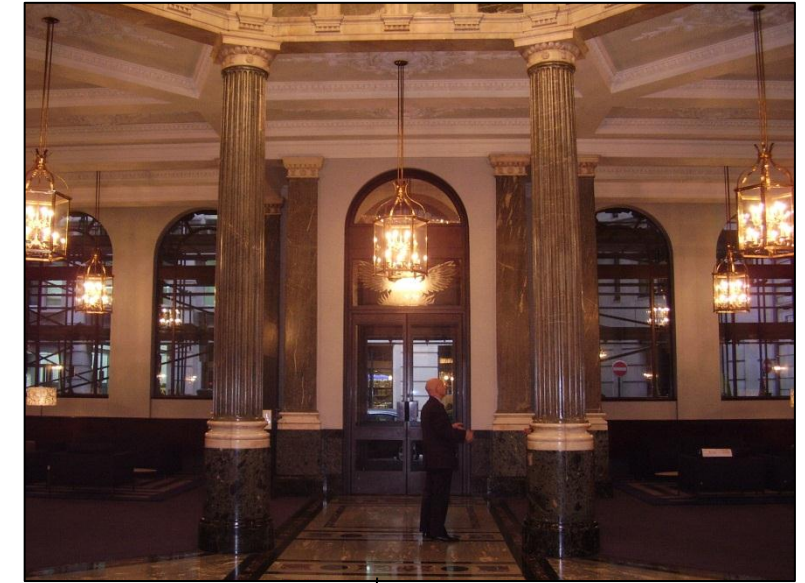
Interior at ground floor, foyer area, where it is proposed to locate contingency propping if required
