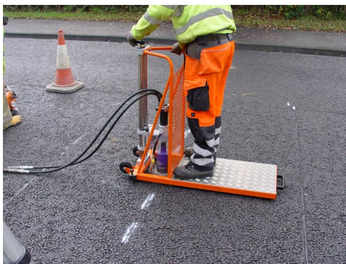
On-street installation of SCOOT detection equipment
