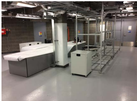
Station operations room test facility at Blackfriars
