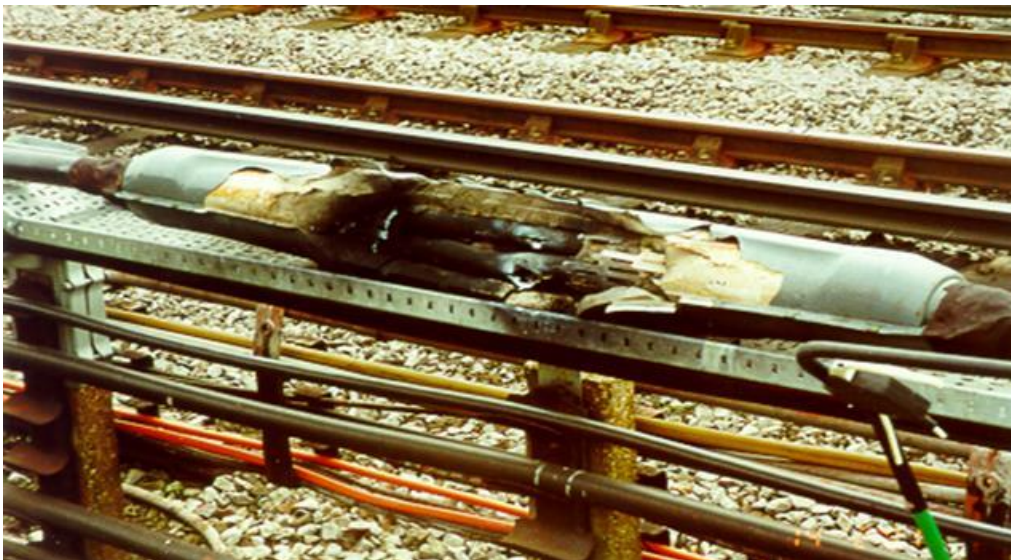
High voltage cable failure
