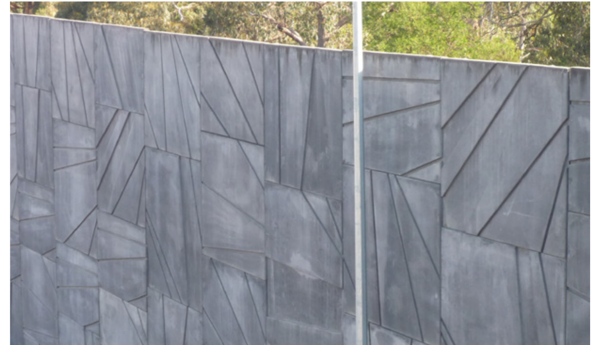
Figure 9.5 Detail of imprinted patterns on environmental / noise barriers
