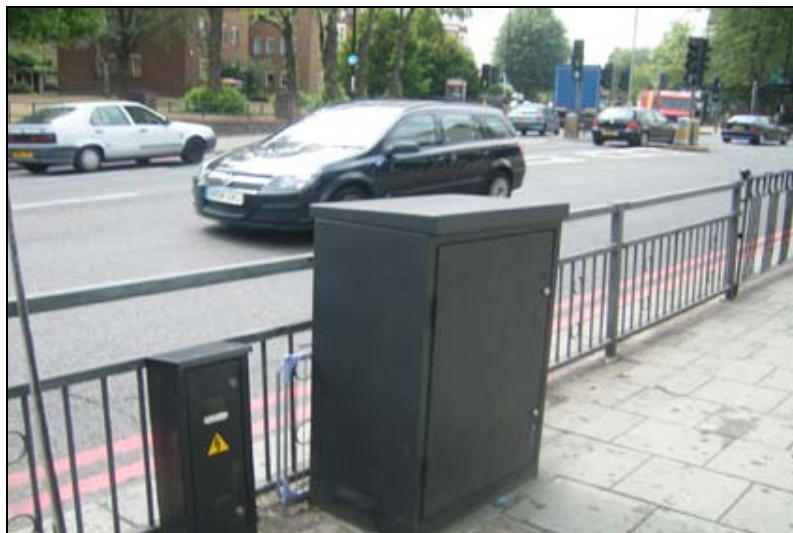
Plate 9.3: Example of control cabinet and feeder pillar
