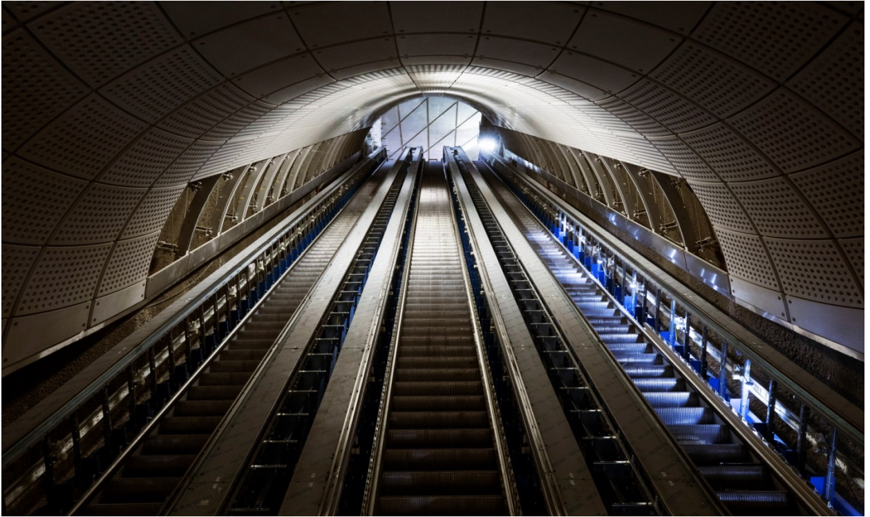
Farringdon station escalators
