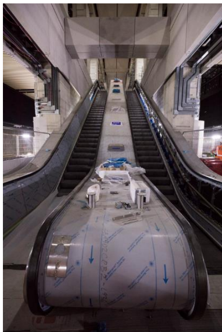
Fig 1. Fully functional escalator bank
