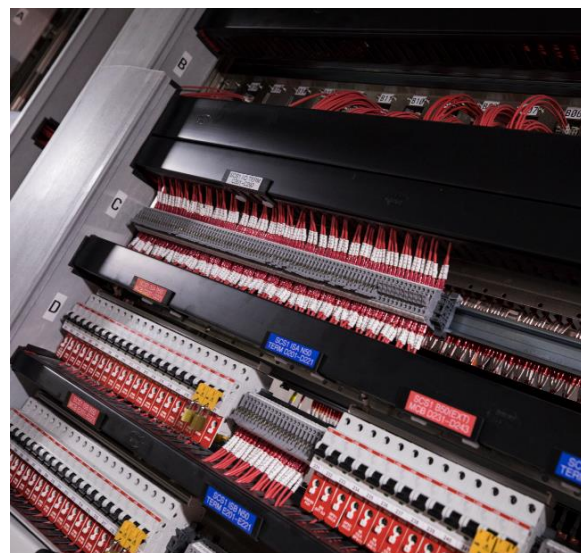
Fig. 4 M&E control panel
