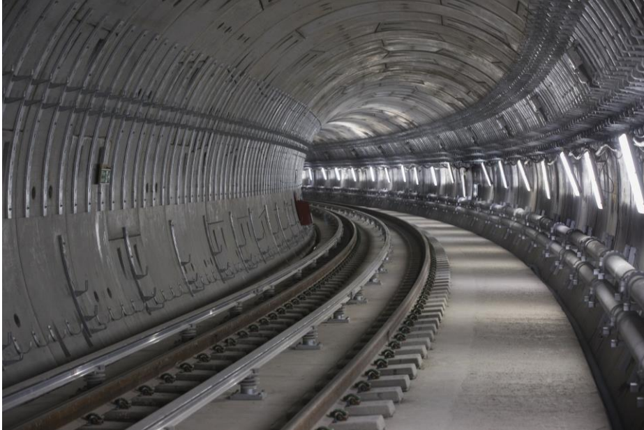
Track installation and tunnel fit out works on going between Kennington Park and Nine Elms Station
