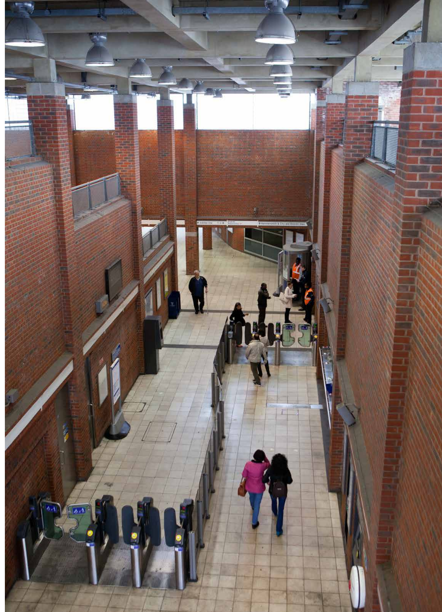
Works progress well on a new ticket hall at West Ham station
