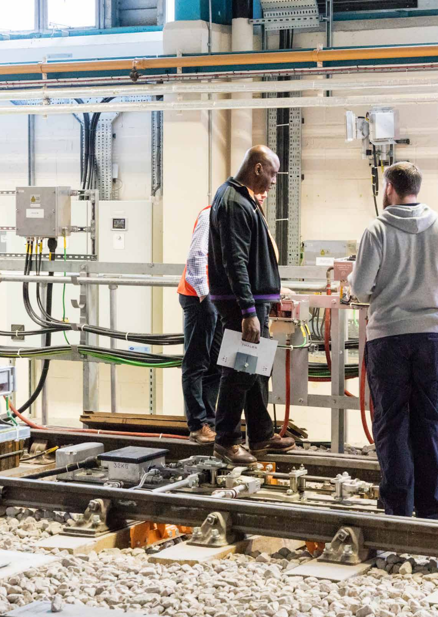
Upgrades to signalling and control ensure safety is paramount
