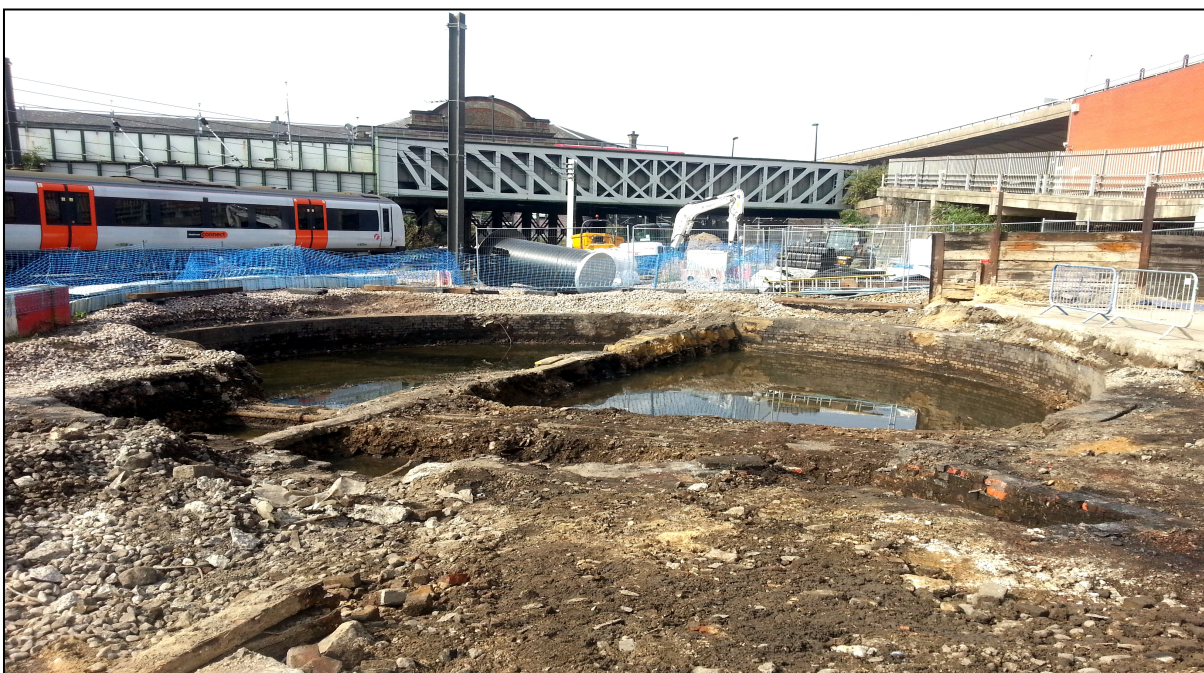
Excavation work at Crossrail's Paddington New Yard site has revealed the remains of Brunel's Great Western Railway
