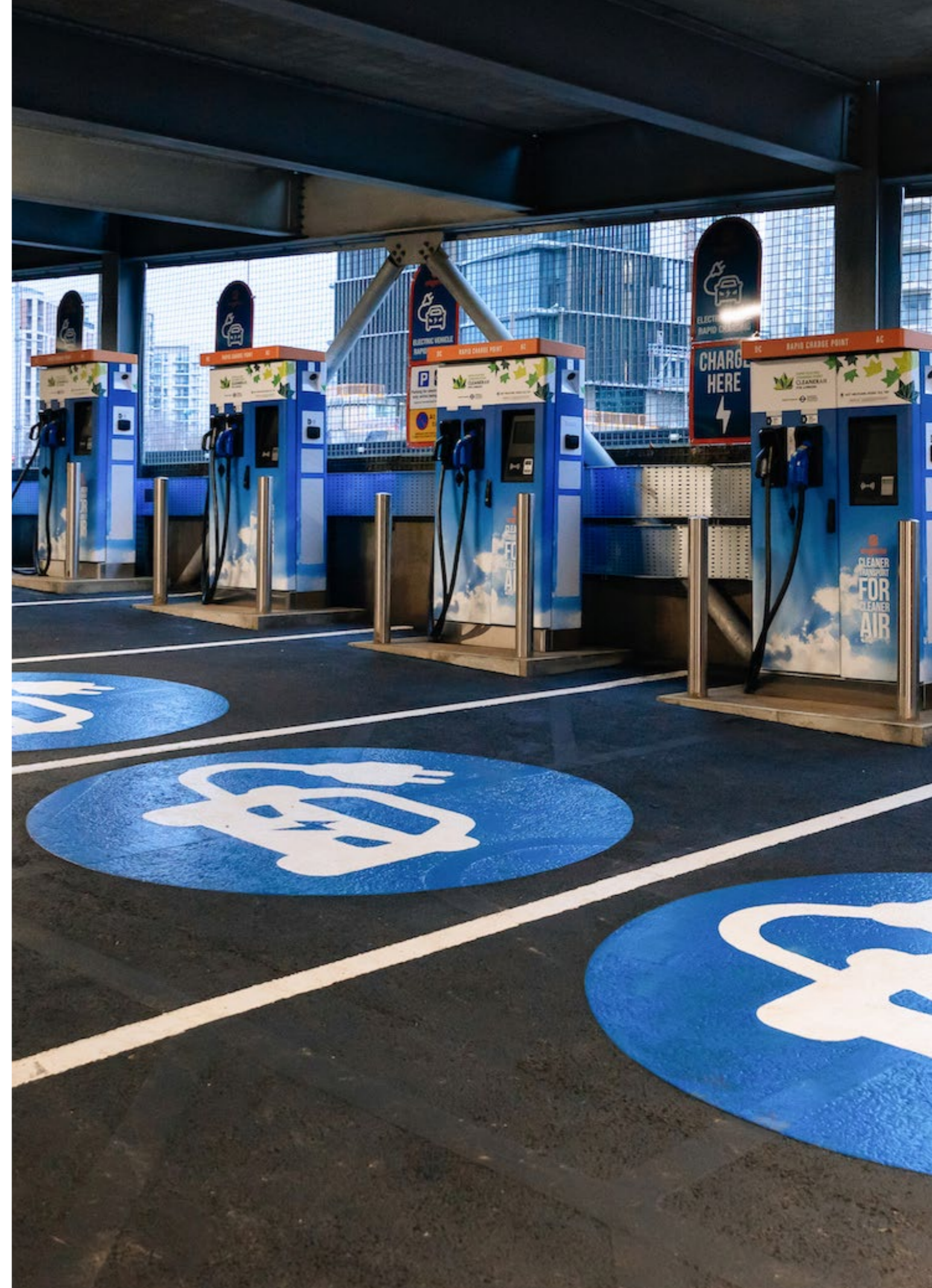
We are installing new vehicle charging points at 100 sites on our roads
