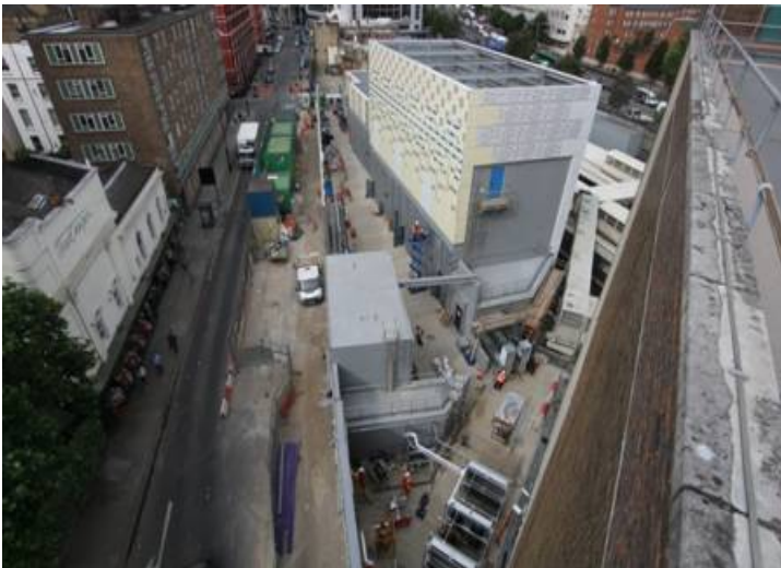
Bulk Supply Point at Griffith House
