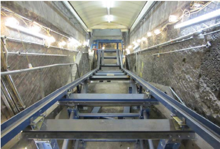
Embankment station installation of temporary works runway system for new escalator delivery route
