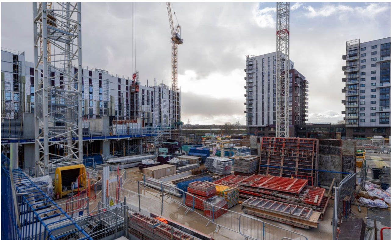
TfL is delivering 350 new homes on the site of a former car park at Blackhorse Road.
