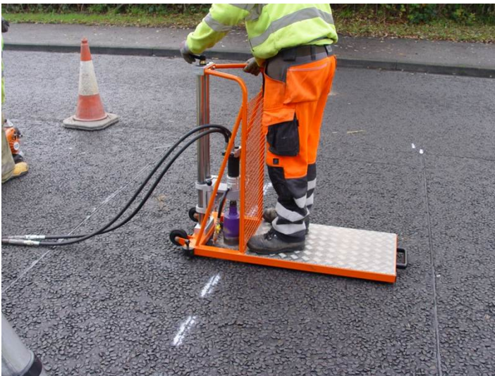
On-street installation of SCOOT detection equipment
