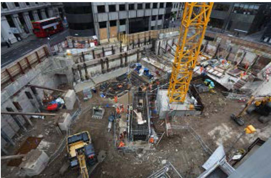
Figure 4 Progress photo: Piling on Whole Block Site (with St Mary Abchurch in background)
