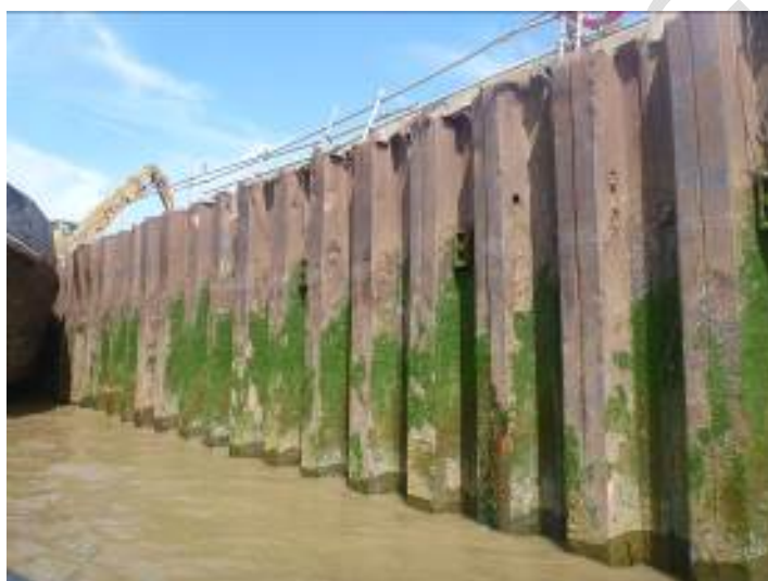
Figure 11: Example of condition of Sheet pile walls of European Metal Recycling upstream frontage.
