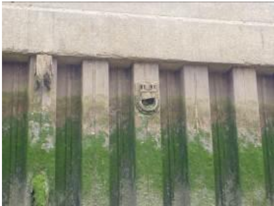
Figure 4 - Broken flap valve on sheet pile wall
