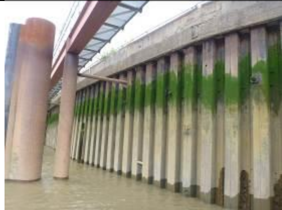
Figure 16 - Steel sheet pile with large diameter fender piles (left) and frame supporting rails for spoil hopper (behind)
