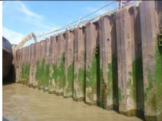
Figure 40 - Steel sheet pile wall with crumple damage to the top of the piles
