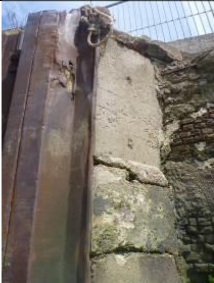
Figure 34 – Damage to concrete interface between sheet pile wall and downstream adjacent masonry wall
