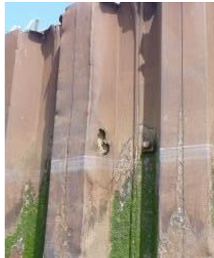
Figure 43 - Localised full-thickness corrosion to sheet piles
