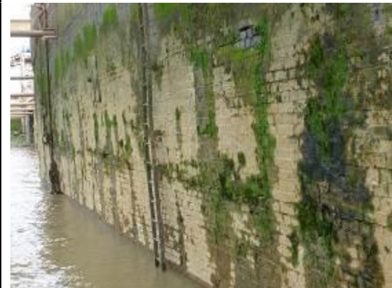
Figure 12 - View of misalignment and bulging in wall
