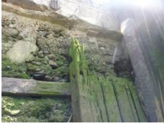
Figure 75 - Timber wall and voids in concrete at intersection with steel sheet piling
