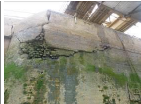
Figure 10 - Section of heavily cracked and unstable masonry at upstream end
