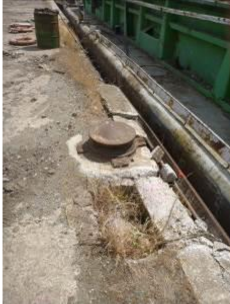
Figure 51 – Damage to coping adjacent to mooring bollard
