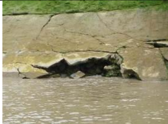
Figure 25 - Void in concrete apron
