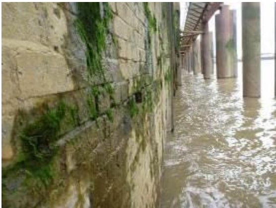
Figure 13 - View of horizontal crack in bed joints mid-height between bed level and anchor height
