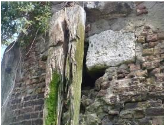
Figure 31 - Voided masonry behind remains of timber fender
