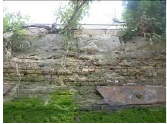
Figure 30 – View of eroded masonry wall with concrete parapet and remnants of steel waling beam.
