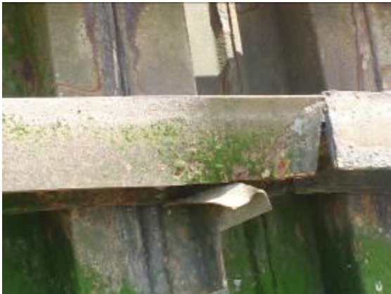
Figure 66 - Impact damage to waling beam
