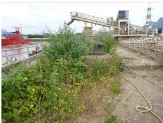
Figure 19 - Vegetation growth behind the raised flood wall
