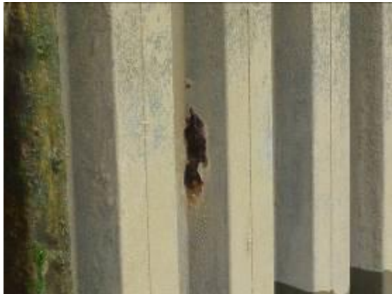
Figure 17 - Localised corrosion, possible Accelerated Low Water Corrosion
