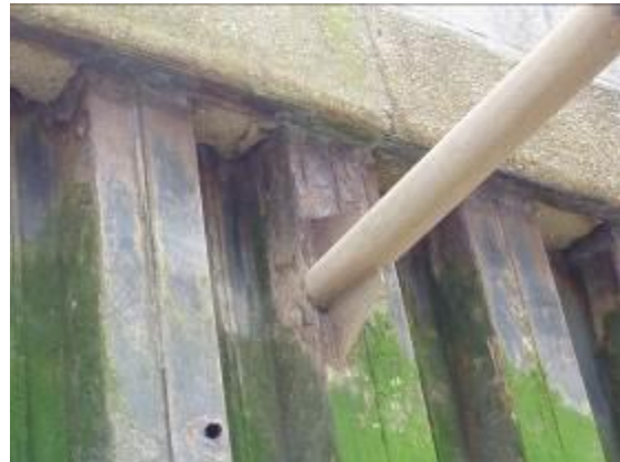
Figure 18 - Welded connection to brace hopper support frame. Elevated corrosion of piles around connection evident
