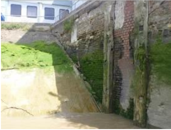
Figure 29 - Interface between masonry wall and masonry abutment. View of large sections of replacement masonry
