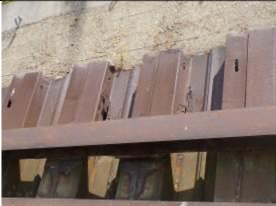
Figure 64 - Full depth corrosion of steel sheet piles with voids in the concrete back fill
