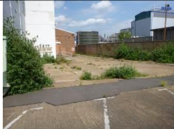
Figure 68 - Cracked and uneven surfacing behind the frontage
