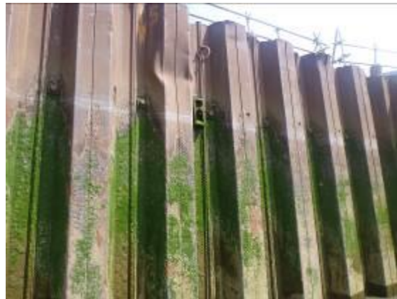
Figure 42 - Impact damage to steel sheet piles
