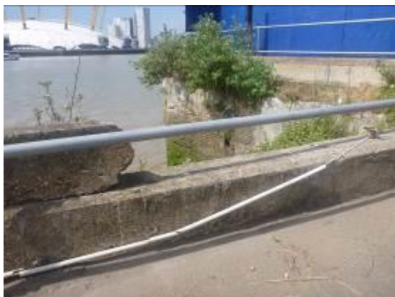
Figure 28 - Missing section of raised concrete parapet
