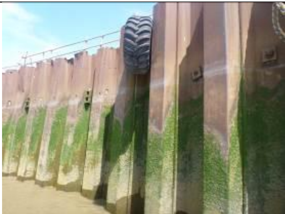
Figure 45 – View of upstream end of asset, showing how the piles have been driven in front of existing frontage
