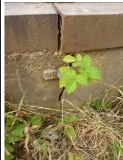
Figure 14 - Crack in concrete parapet with crack monitoring plates
