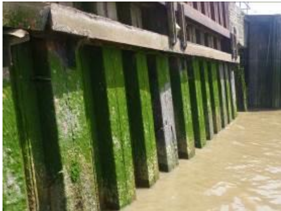
Figure 65 - Steel sheet pile wall with external waling beam. Piles leaning backwards
