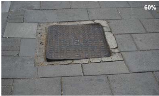
The ironwork is uneven by 20mm
