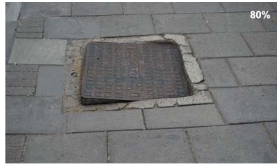
The ironwork is uneven by 30mm
