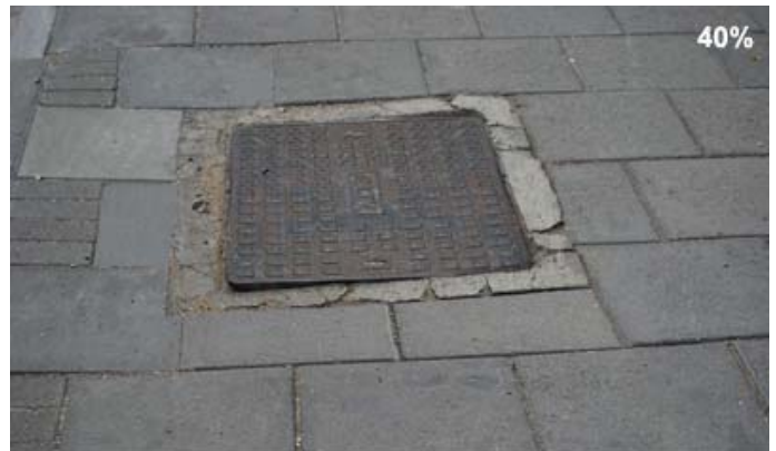
The ironwork is uneven by 10mm
