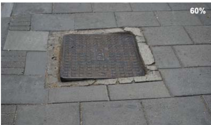
The ironwork is uneven by 20mm
