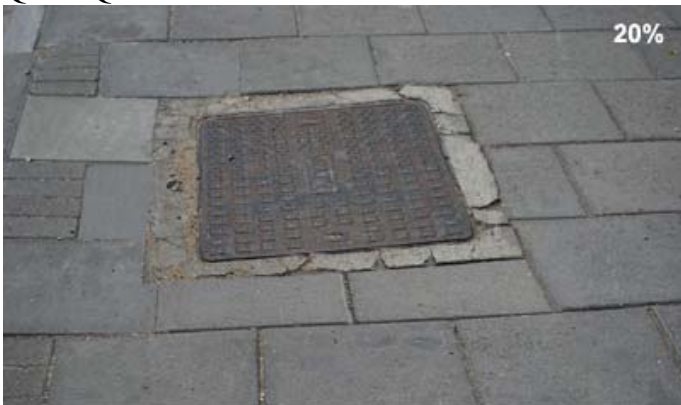
Cracks occurring on the outside of the ironwork
