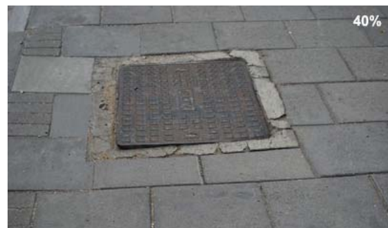
The ironwork is uneven by 10mm
