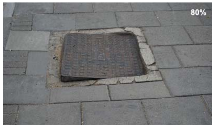
The ironwork is uneven by 30mm
