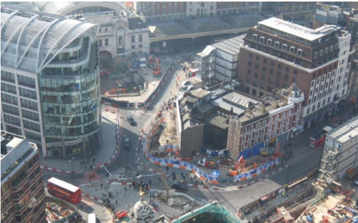
Aerial view of westbound link and south ticket hall worksites at Victoria
