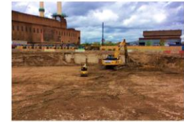
The excavation for the future station is taking place at Battersea. May 2015
