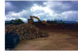
Concrete segregation. May 2015. This shows where we are dividing material in order to recycle and use again on site.
